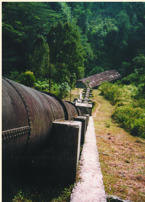
FIGURE 6 The impressive power plant at Malabar (1.5 MW). Though still running, it urgently needs renovation. Hopefully, this historic plant will benefit from the renewed interest in hydropower and remain operational for another century. (Photo by Sven Dervedde)
