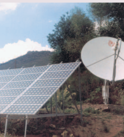
FIGURE 3 A newly established automatic telephone exchange in Pangi Valley, operated by solar batteries. Construction of this installation was a welcome but temporary source of income for the local population. (Photo by Shahnawaz, 1997)
