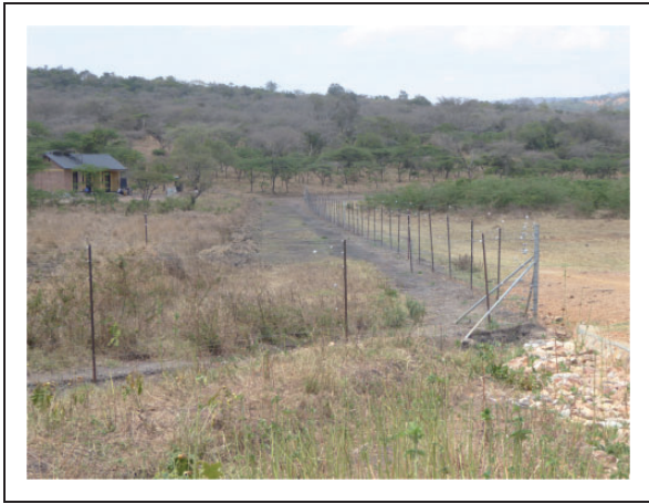
Figure 5. Akagera National Park (Rwanda) Electric Fence, a 2.8 mio $ investment through Rwandan public funds at the start of the delegated management period. Its maintenance, with considerable annual costs, has been assured by the private delegated management partner. This has allowed the re-introduction of Lion and Black Rhino part of an intensified tourism program (photo by Paul Scholte, 2016).
