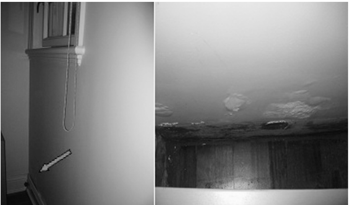
Fig. 3. Effect of high air humidity in basement.
