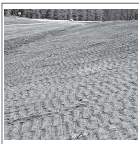
Figure 5. Trackwalking is often used to increase slope stability, but will compact both surface and subsurface soils.
