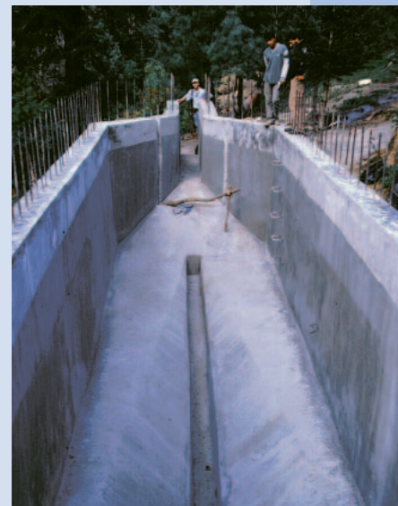
FIGURE 3 Desilting tank in Kothi. The tank ( 34 \times 2.5 \times 1.5 m), made of reinforced concrete, desilts water on its way to two 100-kW turbines. (Photo by author)
