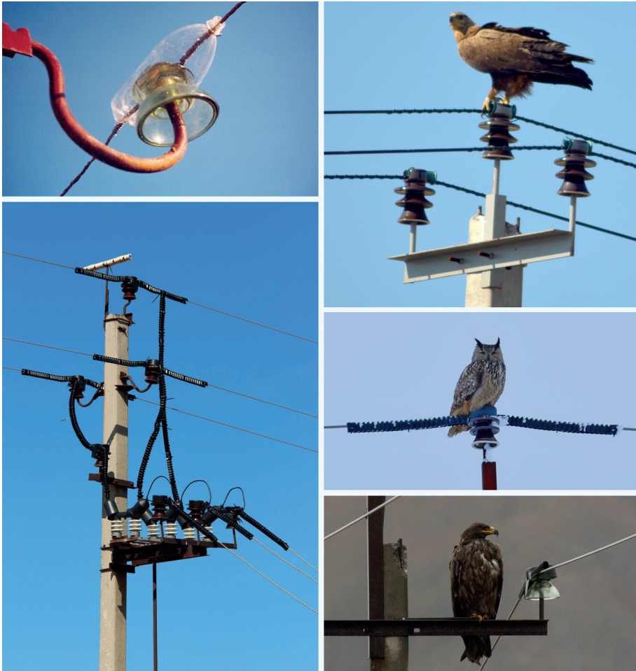
FIG. 6.— Bird Protection Devices (BPDs) designed specifically to fit the 6-10kV electric system in Kazakhstan and southern Russia. Top left: A plastic bottle used before BPDs were available in the region (photo: Adrey Saltykov from Medzhidov et al. , 2005). Top right: a Steppe Eagle Aquila nipalensis perched on insulated wire in Southern Ural, Russia (photo: Igor Karyakin). Centre right: A Eurasian Eagle-Owl Bubo bubo perched on a conductor cover in the Kalmykia, Russia (photo: Gennadiy Erdnenov). Bottom left: BPDs on conductors, jumpers, and equipment on a switch pylon (photo: EcoNIOKR). Bottom right: Steppe Eagle perched adjacent to a conductor fitted with a cover in Altai, Russia (photo: Márton Horváth).
