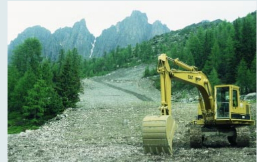
FIGURE 4 Clearing forests to build ski runs conflicts with the need to maintain the protective functions of forests. (Photo by Pier Carlo Zingari, 1988)
