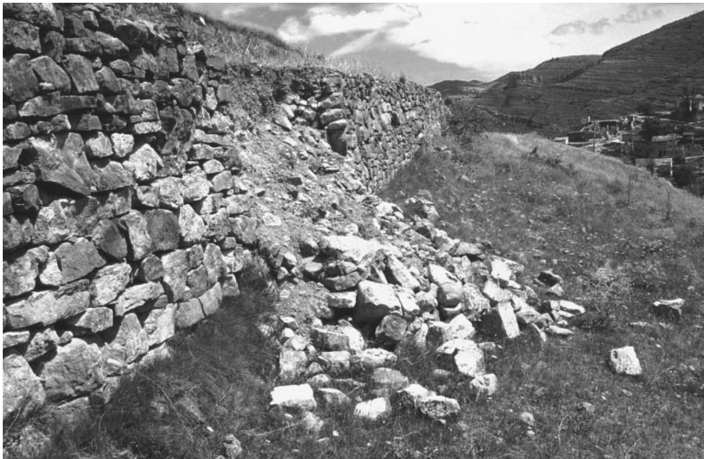
FIGURE 5 Collapse of a terrace wall at the foot of a hill near a village resulting from hydrological pressure higher up (Soto en Cameros, Leza Valley). Fields in this gently sloping area were only abandoned within the last 10 years. (Photo by L. Ortigosa)
