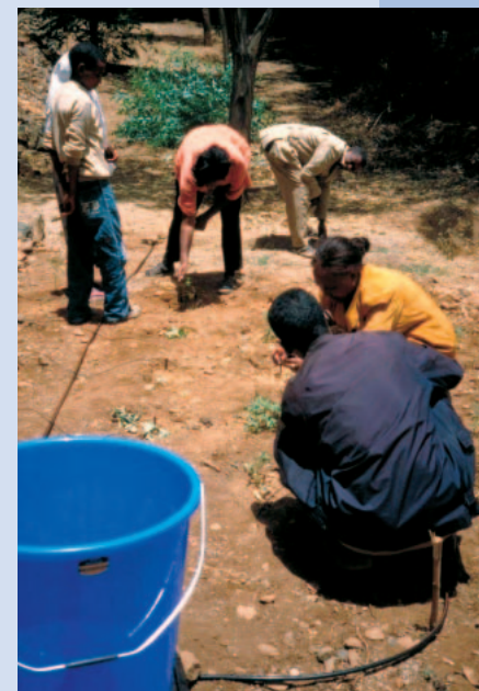
FIGURE 5 Successful use of drip irrigation depends on support from specialists for installation and maintenance. (Photo by Brigitta Stillhardt)
