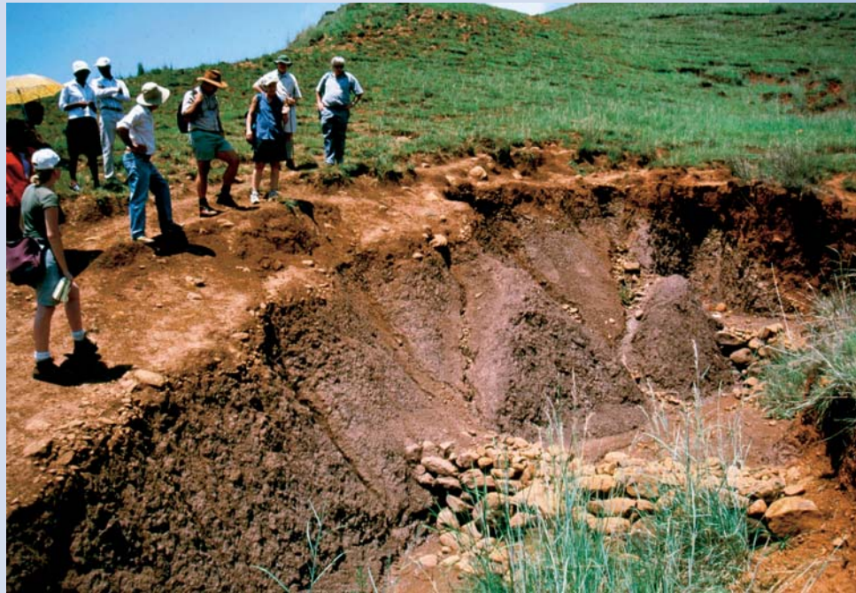
FIGURE 4 Gully erosion near Mnweni, in the Kwa-Zulu/Natal part of the study area. The local community has undertaken reclamation work to halt erosion. (Photo by Greig Stewart)
