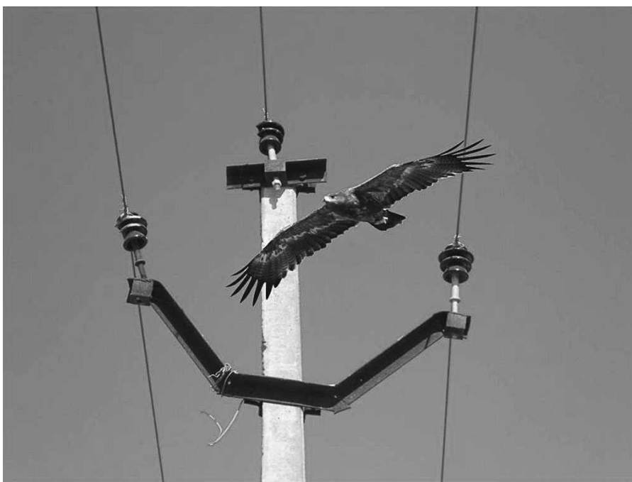
Figure 1. Typical 11-kV concrete pole with a grounded metal cross-arm. A Steppe Eagle ( Aquila nipalensis ), a common raptor in Rajasthan, India, with a wingspan of 165–190 cm, provides a reference for relative size.
