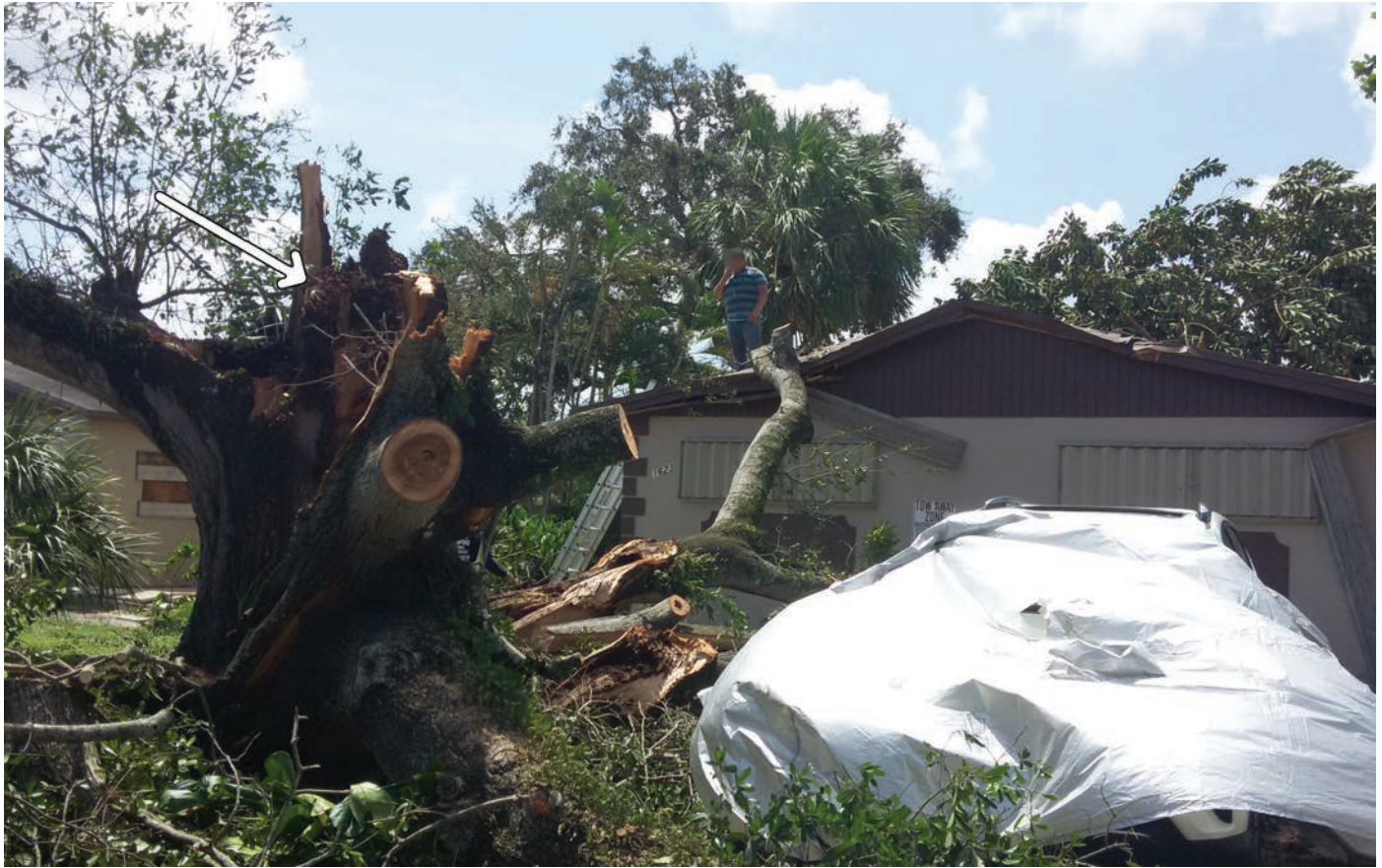
Fig. 10. Large oak tree hollowed out by Coptotermes gestroi , with presence of carton at the center of the tree (arrow), and property damage resulting from the tree structural collapse during hurricane Irma (Sep 2017)
