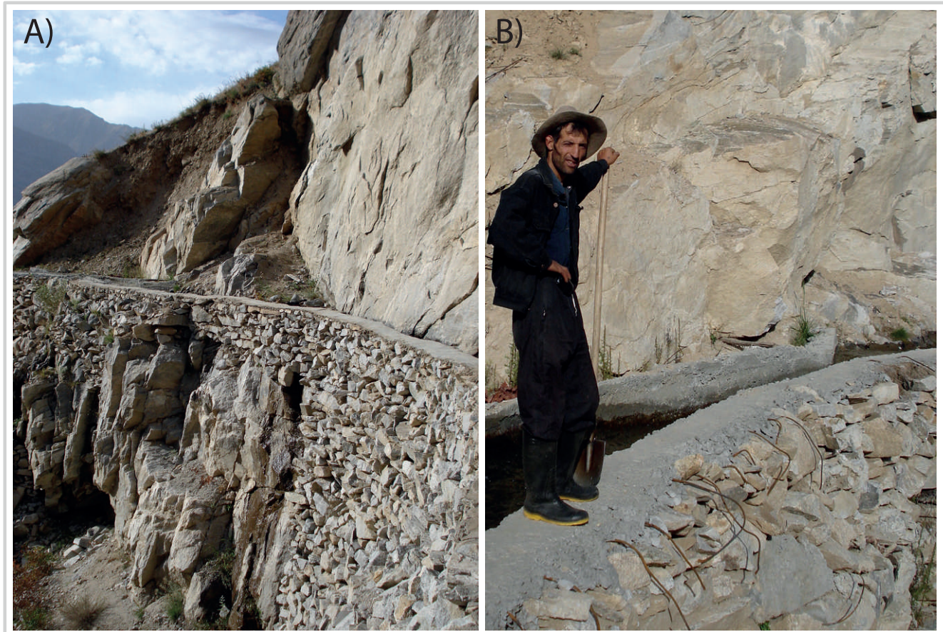
FIGURE 3 (A) Canals are often situated on steep slopes; (B) they require a great deal of maintenance. (Photos by Lisa Bossenbroek)
