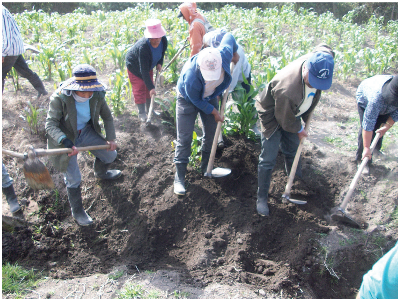
FIGURE 2 Resettlers in a collective work party ( minga ) rebuilding an irrigation network in the high-risk zone at the foot of the volcano. Minga is one of many forms of cooperation and reciprocity practiced in the area. (Photo by A. J. Faas)
