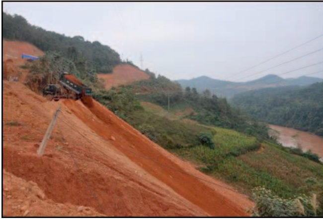
Figure 5. Road construction and disposal of debris over the edge of the road and the impact on the local river; the river is the same color as the earth being dumped. Lang Son Province, Vietnam. Photograph by Arthur Bogan. November 11, 2012.
