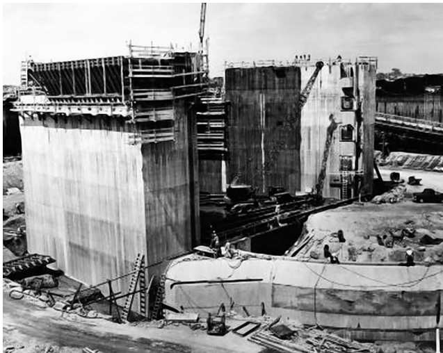
Figure 15. Construction of the sector gatehouse, New Bedford barrier, 1964. The structure in the lower right is a guide for the gate rollers and also contains a tunnel through which the gate operators can walk under the channel (photograph courtesy NAE).
