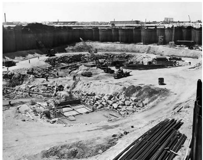
Figure 14. Sector gate foundation work within protective cofferdam, New Bedford harbor, Massachusetts, 5 May 1964 (photograph courtesy NAE).
