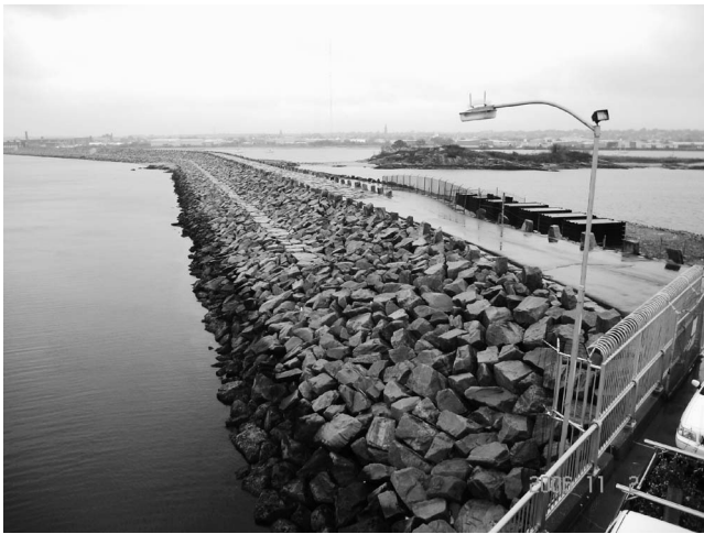
Figure 11. New Bedford dike, view west from gate control house, 2 November 2006 (photograph by A. Morang)
