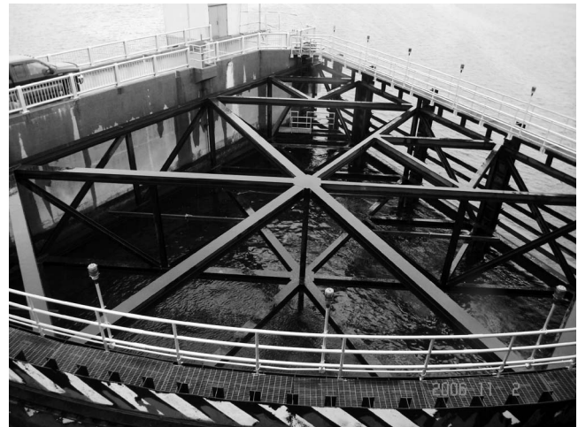
Figure 16. West side sector gate in rest position, New Bedford hurricane barrier, 2 November 2006. The pivot is at the upper center of the photograph, and the ship channel is to the right. Silt builds up in the basin and must be flushed with compressed air. The gate is operated by a 25 hp electric motor (photograph by A. Morang).
