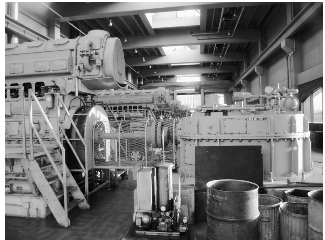
Figure 26. Diesel engines and pumps in Charles River Dam, 1 November 2006 (photograph by A. Morang).
