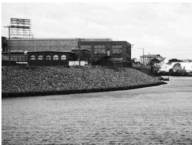
Figure 20. Hurricane surge barrier, west bank of Pawcatuck River, Stonington, Connecticut (photograph by A. Morang, taken from Westerly, Rhode Island).
