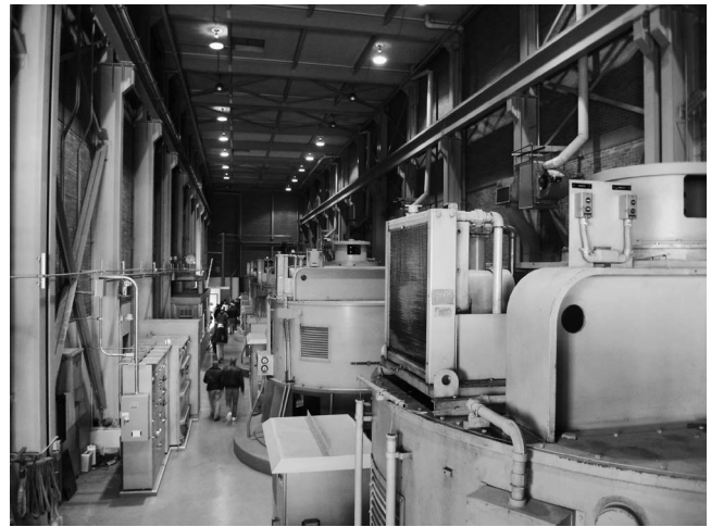
Figure 8. Fox Point pump house, 4 November 2006 (photograph by A. Morang).
