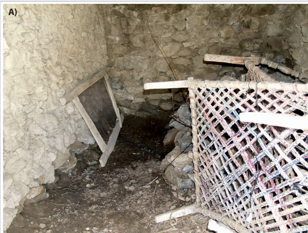
FIGURE 3 (A) Seepage inside a house located below an irrigation channel; (B) cracks in a house as a result of heavy seepage. (Photo A by Jawad Ali; photo B by Muhammad Asad Salim)
