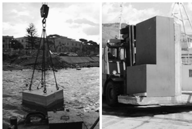
Figure 3. (a) The caisson utilized during the experiment RC-2001. (b) One of the nine modules constituting the absorbing breakwater of the experiment RC-2005.
