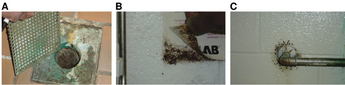
Fig. 1. German cockroaches and cockroach feces in conventionally treated schools. (A) German cockroaches infesting a floor drain. (B) Heavy German cockroach infestation and fecal smears behind a poster in the kitchen. (C) German cockroaches infesting a wall plate beneath the kitchen sink. (Online figure in color.)
