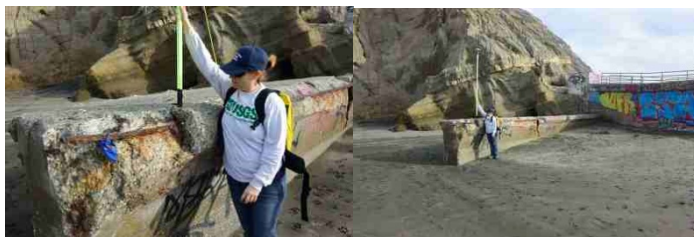
Ground Control Point 116: Corner of northern outlet structure at base of cliffs.
