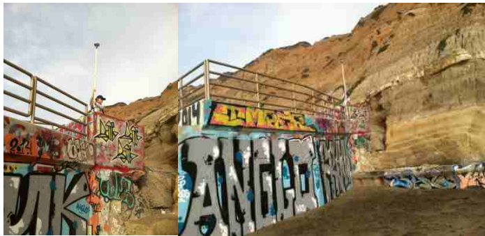
Ground Control Point 122: Southern corner of upper portion of the northern outlet structure.
