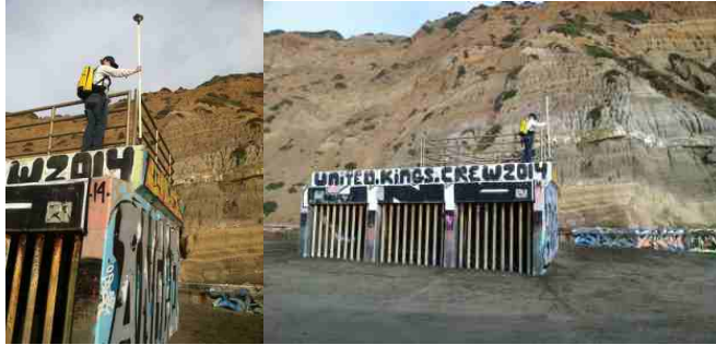
Ground Control Point 121: Southern corner of seaward portion of the northern outlet structure.
