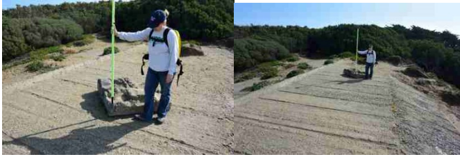
Ground Control Point 35: Northern corner of concrete block on roof of the northernmost battery of the "Davis Group."
