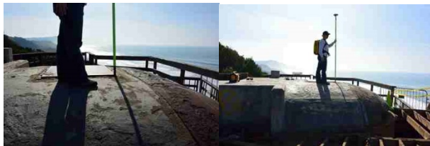
Ground Control Point 14: Northwestern corner of a metal plate on the southernmost small battery in the “Funston Group”
